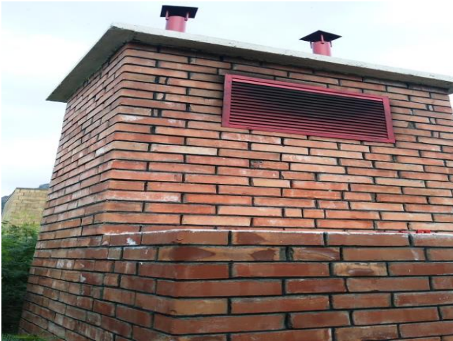
Incinerator at 30 November School,, Al-Mafalis area, Hayfan, September 10, 2022
