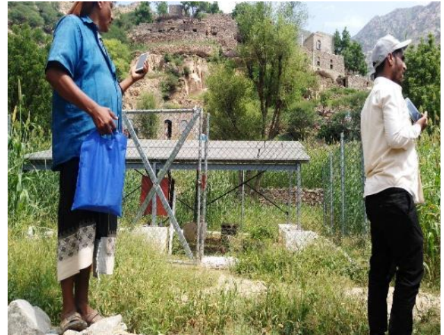
Solar panel for AlSabad water project, Hayfan, captured by MEAL Center field staff, September 11, 2022
