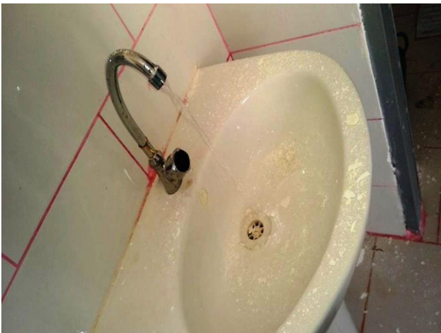
Hand washing facilities are functional and water is accessible at 22 May school, As Silw district, captured by MEAL Center field staff, September 13, 2022
