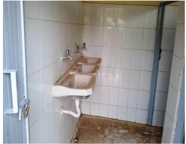
Latrines at 30 November School,, Al-Mafalis area, Hayfan, captured by MEAL Center field staff, September 10, 2022
