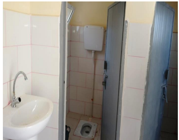
Latrines at 22 May school, As Silw district, captured by MEAL Center field staff, September 13, 2022
