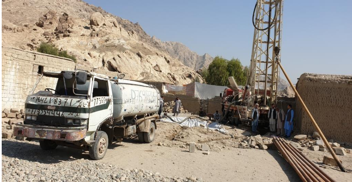
Photo 9: The view of a well drilling by Rotary Rig Machine in Daman
