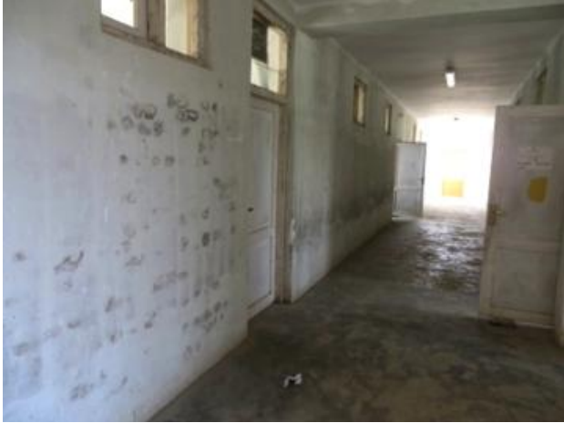
Figure 3: Unpainted walls inside the building.
